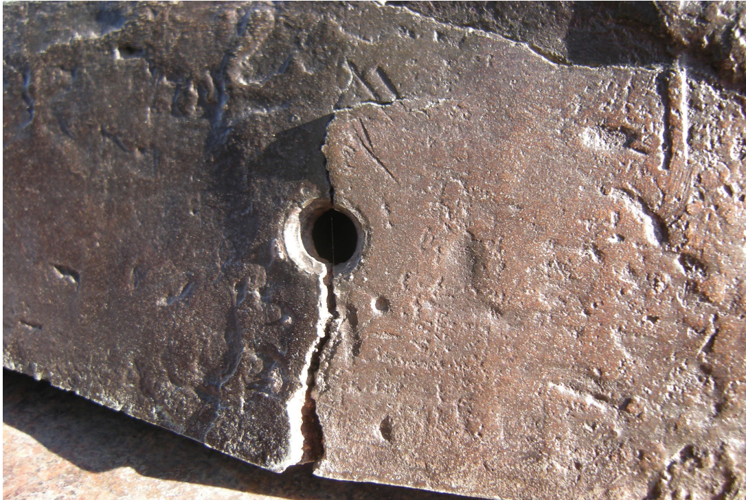
Fig. 3. Detail of damage from rust jack expansion of internal support
