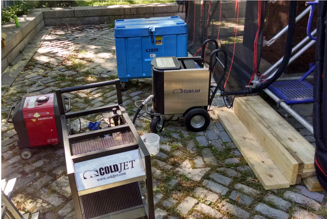
Fig. 12. Dry ice blasting system with aftercooler in foreground
