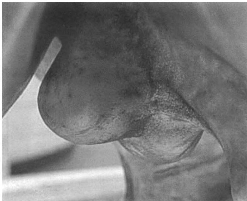
Figure 18. Detail of spot corrosion on the gilded surface of the Quadriga, underside of a horse, 1999.
