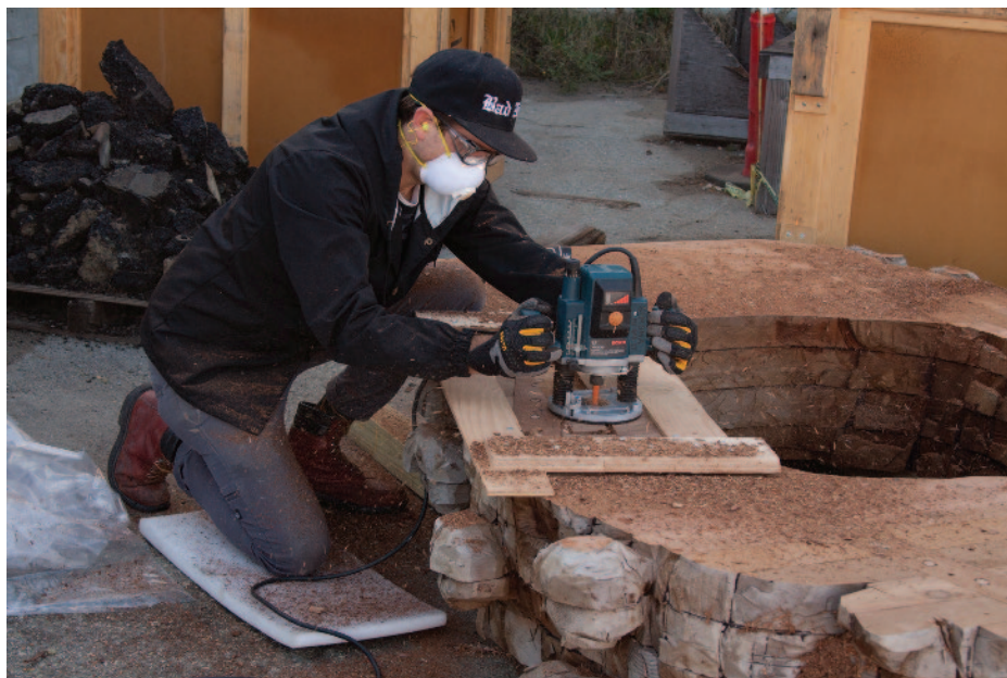
Fig. 9. Routing out a crossbeam that was damaged by the previous mount. The damaged area was then replaced with a new cedar crossbeam (Courtesy of Ursula von Rydingsvard, Photograph by James Gouldthorpe)
