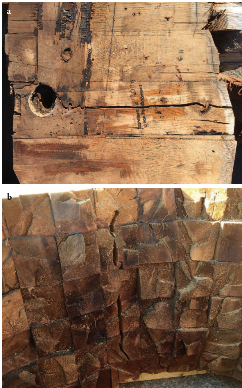
Fig. 4a. Crack caused by previous mount as viewed from above; 4b. View from the side (Courtesy of Ursula von Rydingsvard, photographs by Emily Hamilton)
