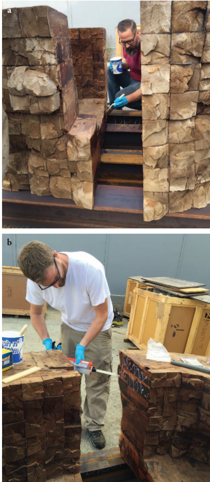
Fig. 5a. Brush application of Prime-A-Trate to separated sections; 5b. Application of Flex-tec HV epoxy (Courtesy of Ursula von Rydingsvard, photographs by Emily Hamilton)
