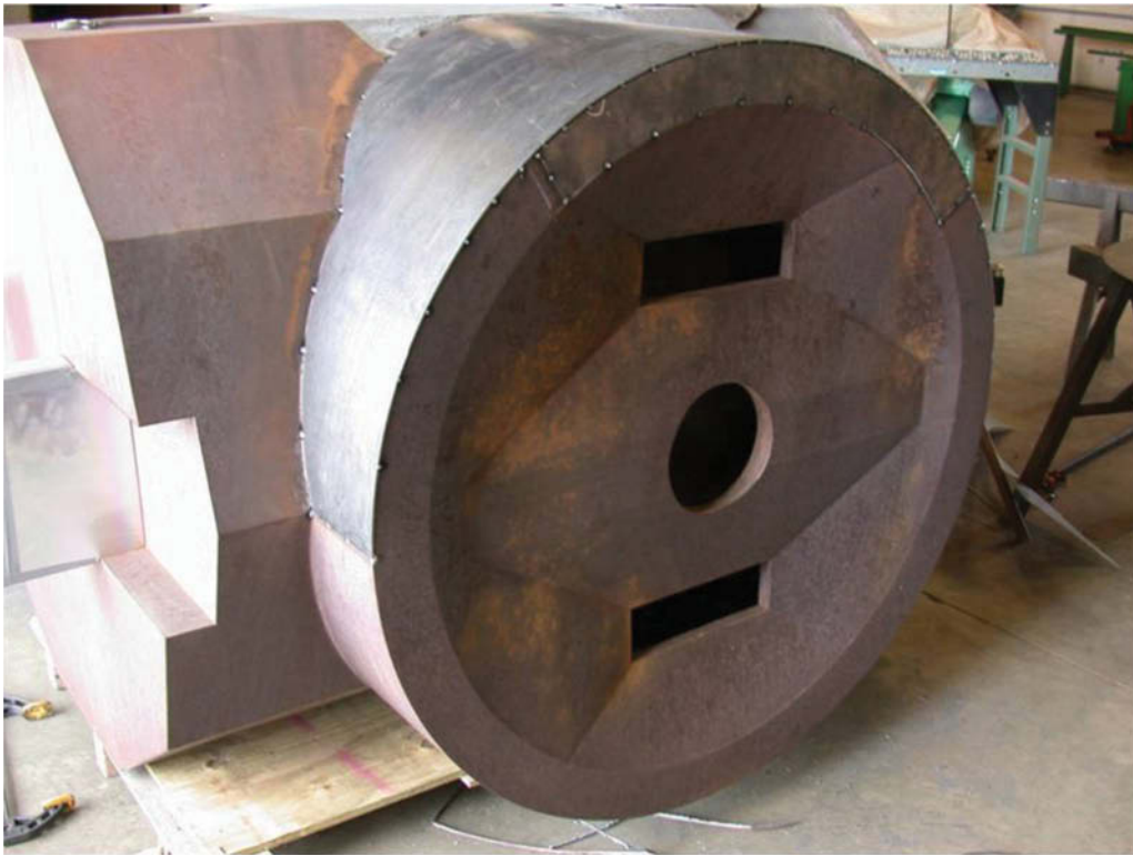
Fig. 19. New sections of COR-TEN steel tack welded in position on the Saint Louis Plug (Courtesy of Russell-Marti Conservation Services, Inc.)
