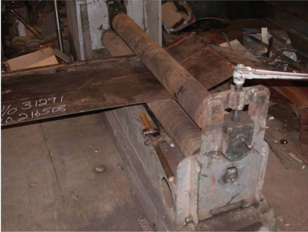
Fig. 18. Rolling the new section of COR-TEN steel to the exact curvature of the original (Courtesy of Russell-Marti Conservation Services, Inc.)
