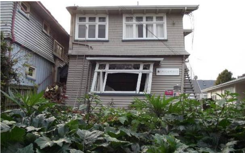
Fig. 4 Damage to wooden structures.
